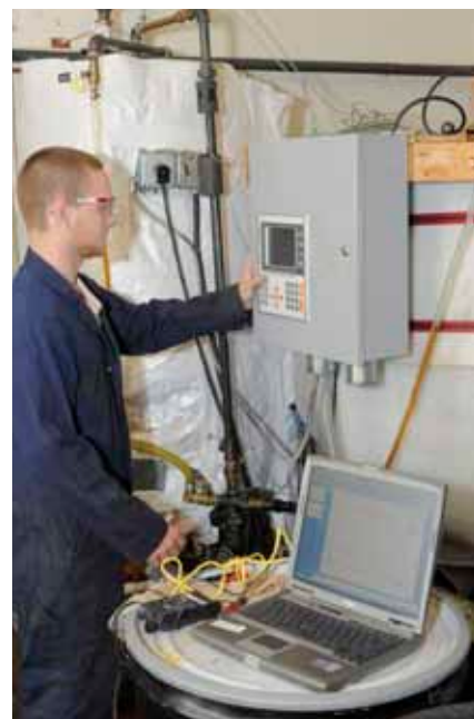
Simple operation with a B&R Power Panel.
